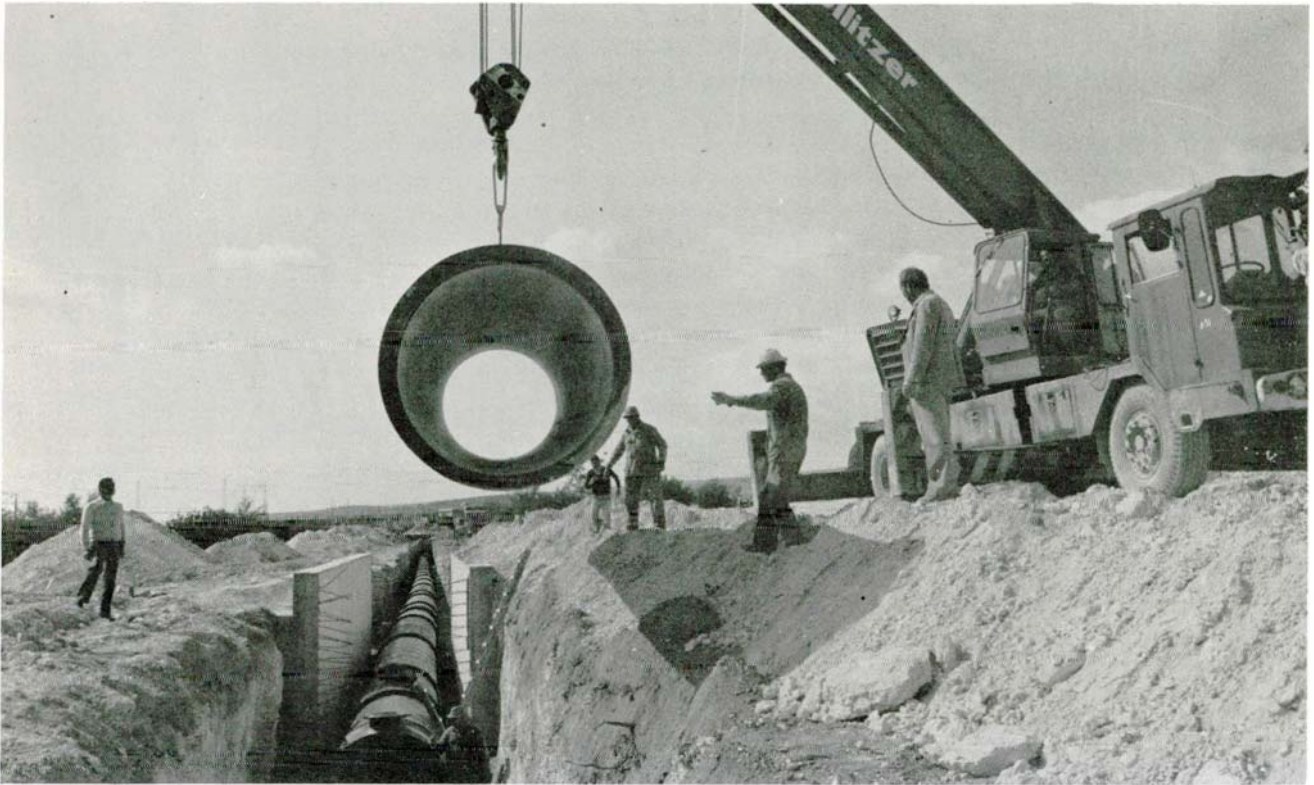
Southern Conveyor Project. Installation of part of main conveyor to facilitate EAC structures along Limassol by-pass at Ayia Phyla. WDD Photo E16-12. (21.2.84)
