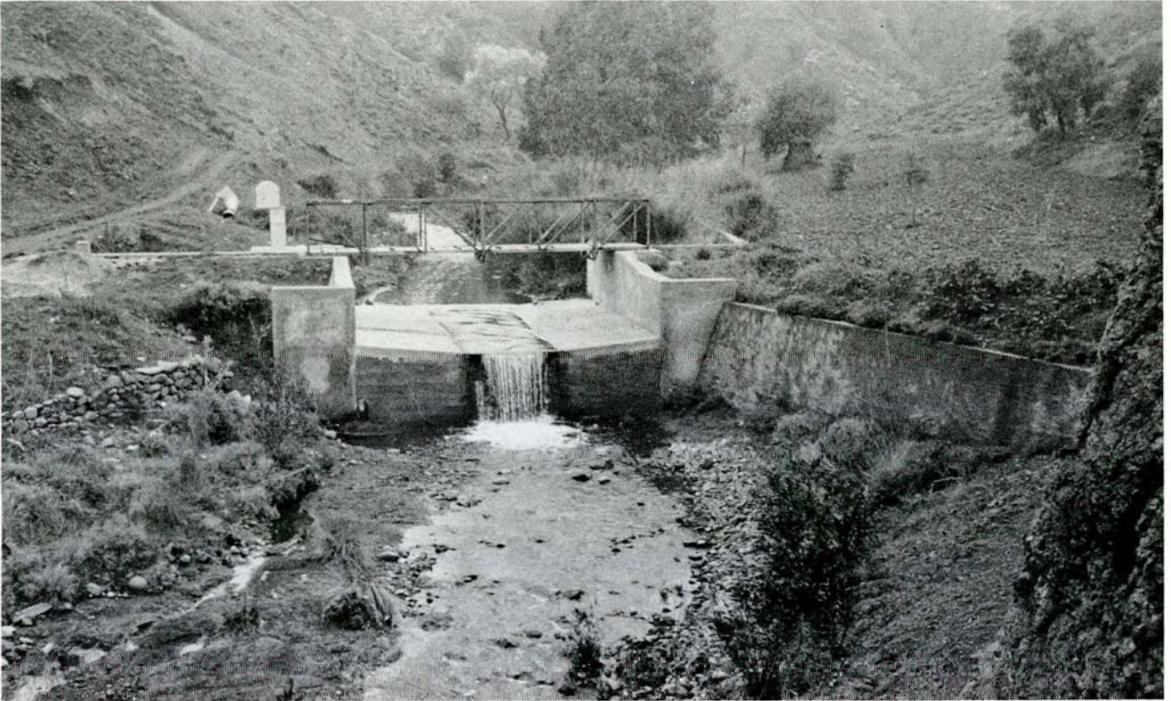
Pedhieos river. Flow gauging station on Ayios Onouphrios stream improved in summer 1984. WDD Photo B91EN-5 (12.2.85).
