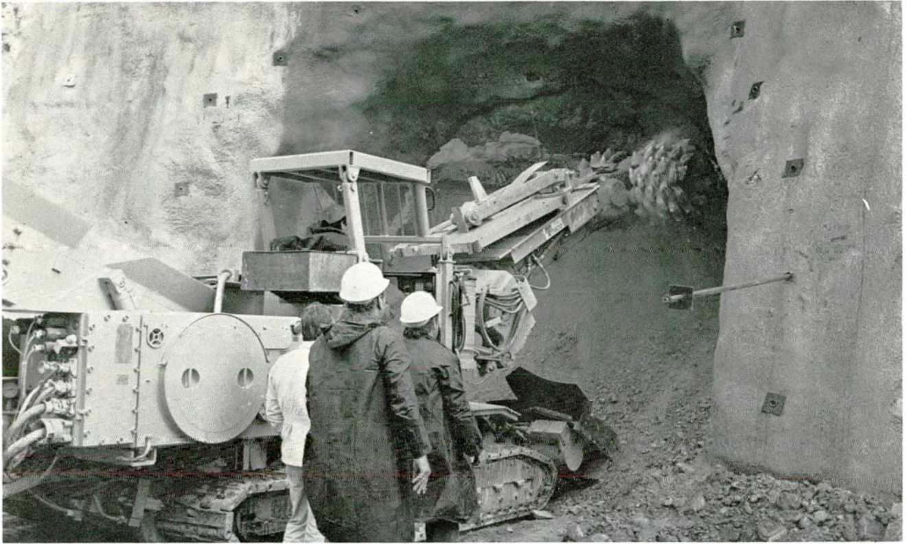
Kouris Dam. Upstream portal of diversion tunnel being excavated by Alpine Miner AM75. WDD Photo E72-7 (10.11.84)
