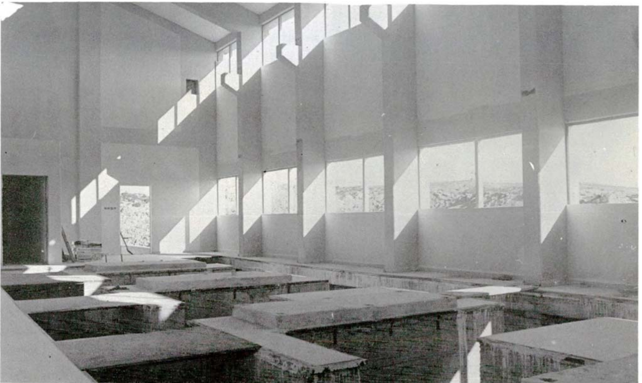
Tokhni Pumping Station with the four floor level pump plinths ready for pump and motor installation. WDD Photo E75-11 (5.12.84).
