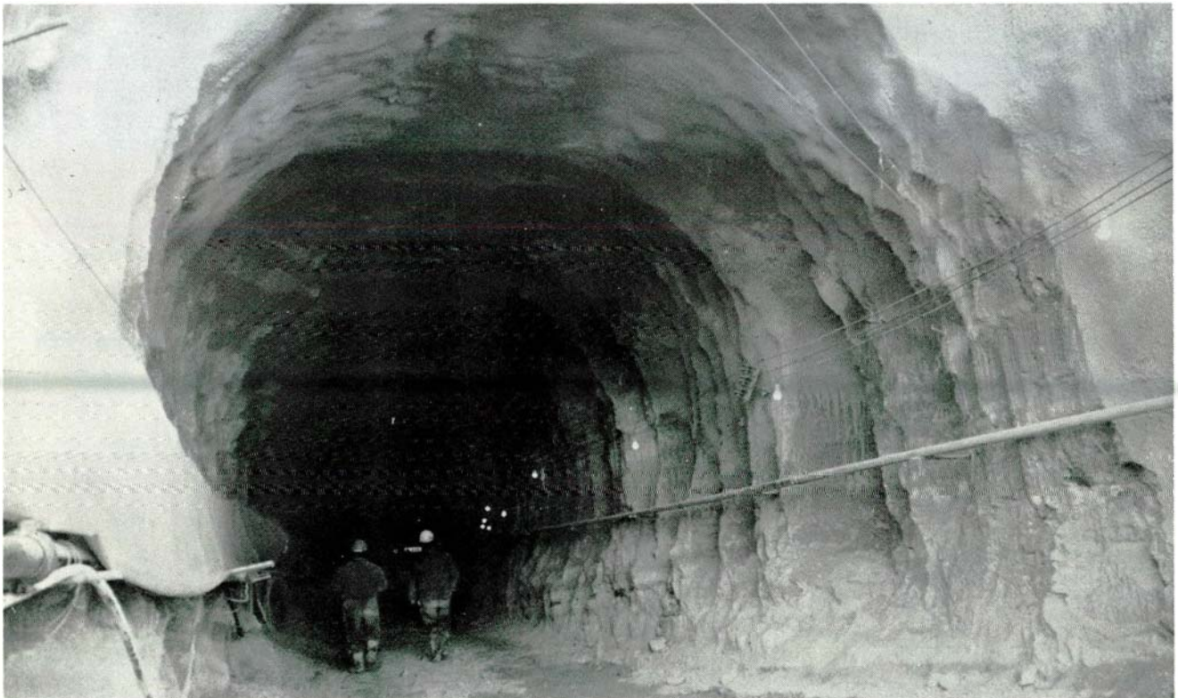
Kouris Dam. Excavated part of the diversion tunnel. Upstream section. WDD Photo E78-3. (17.12.84)
