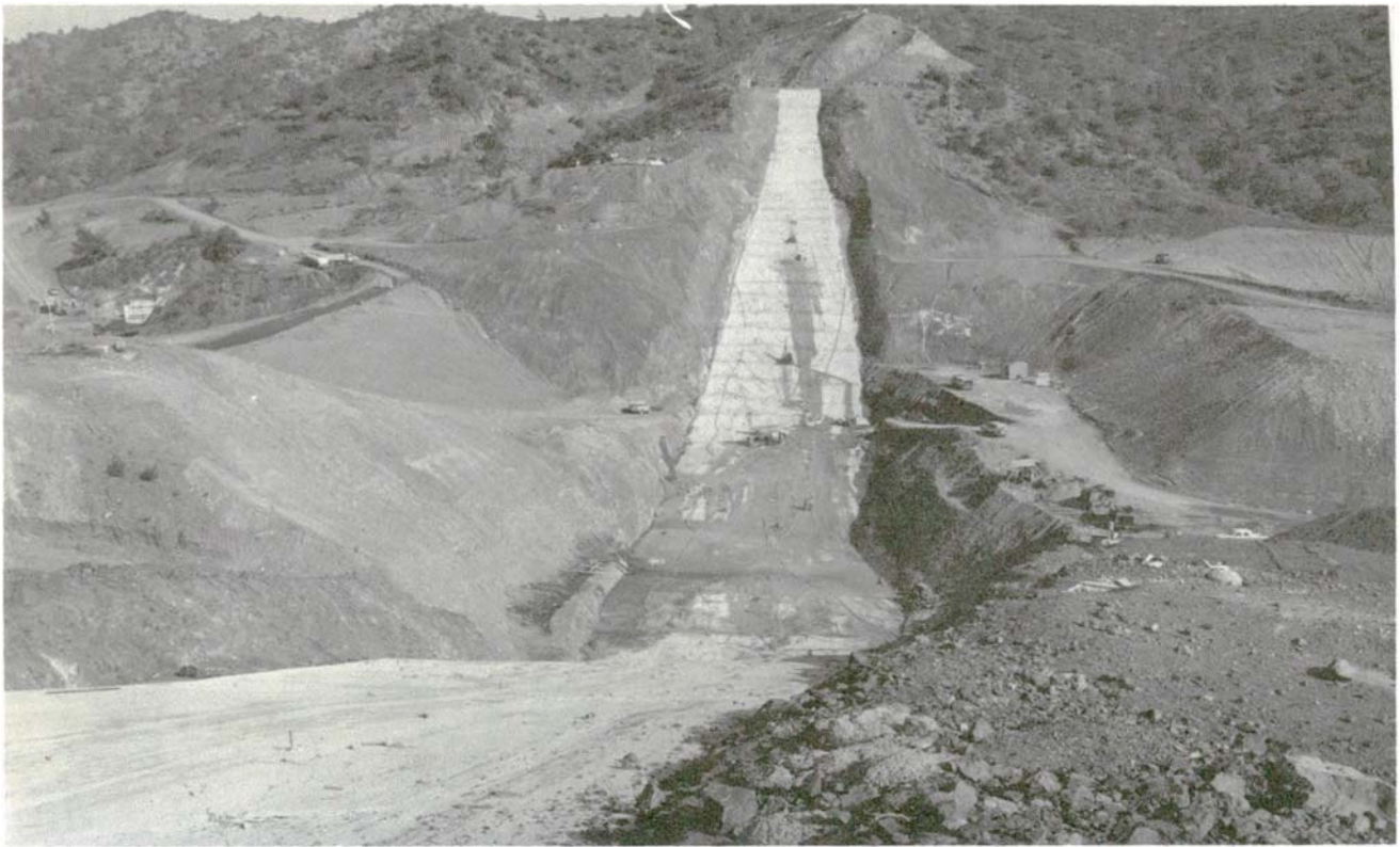
Dhypotamos dam. Cut-off trench excavation and left abutment viewed from top of right abutment. WDD Photo D94-7, 6.12.83
