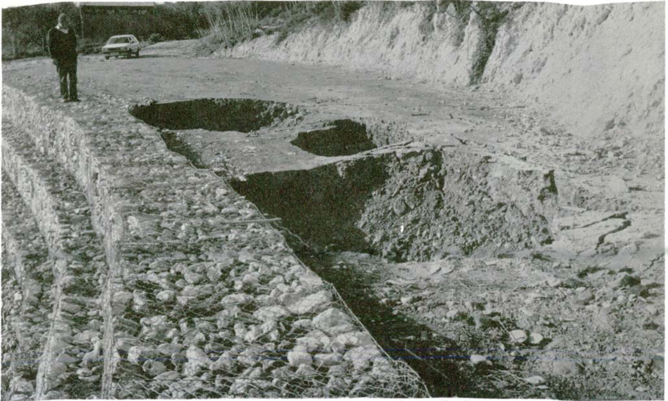
New sinkholes developed after the construction of the protection wall in the Maroni River. WDD Photo E4-11, 4.1.84.
