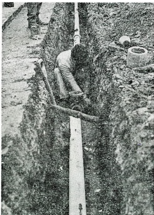
Laying of New Water Supply Pipelines within the Walled City of Nicosia
