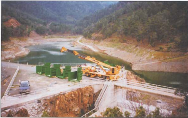
Installation of the fusegates at Xyliatos dam. Each fusegate weighs about 2 t.
